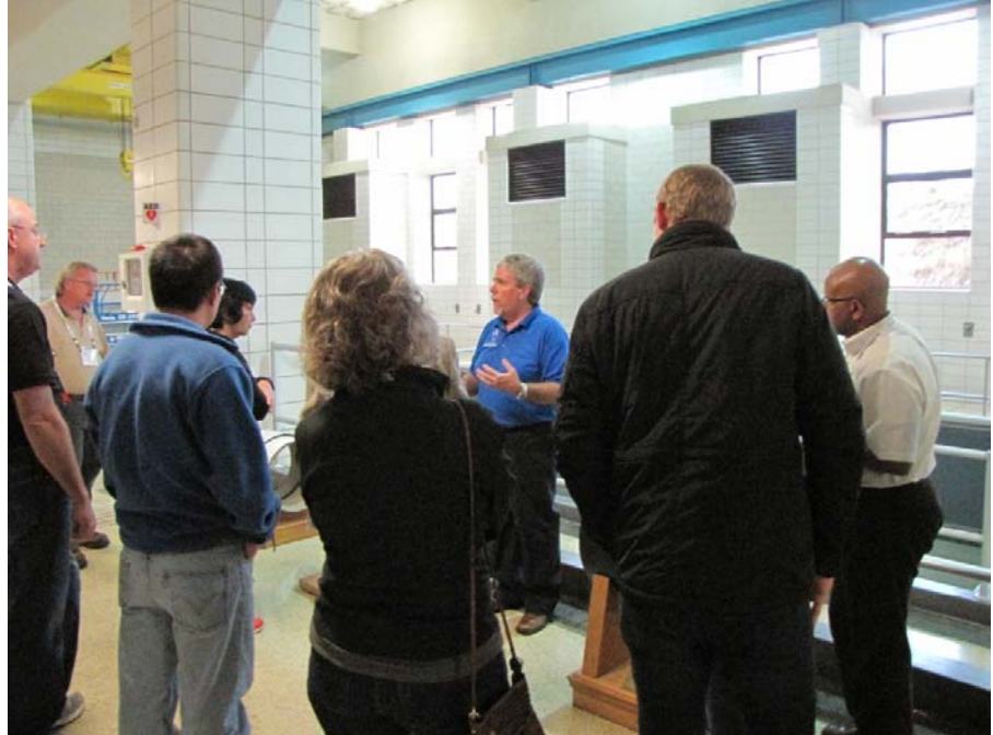
McGhee describing the different types of pipes and valves in DWC's system
